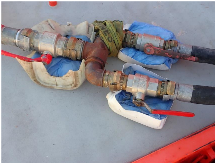
Figure 12. Leak containment precautions at a connection point in the fuel line from ship to bulk fuel storage tanks on Lion Island
