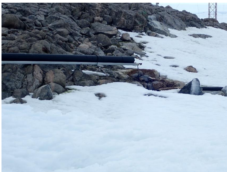
Figure 29. Waste water outlet from summer dormitory in lower station area
