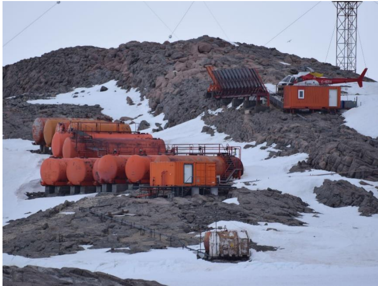
Figure 13. Annual bulk fuel tanks in the lower station area
