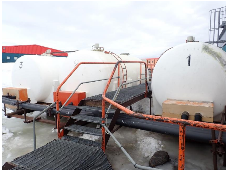
Figure 8. Fresh water tanks in the upper station area
