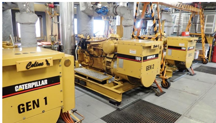
Figure 9. Diesel generators in the main powerhouse
