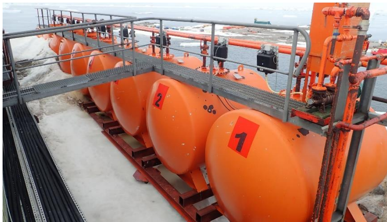
Figure 14. Bulk fuel tanks in upper station area
