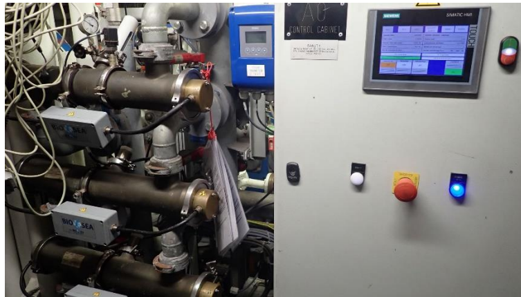
Figure 47. Ballast water treatment unit
