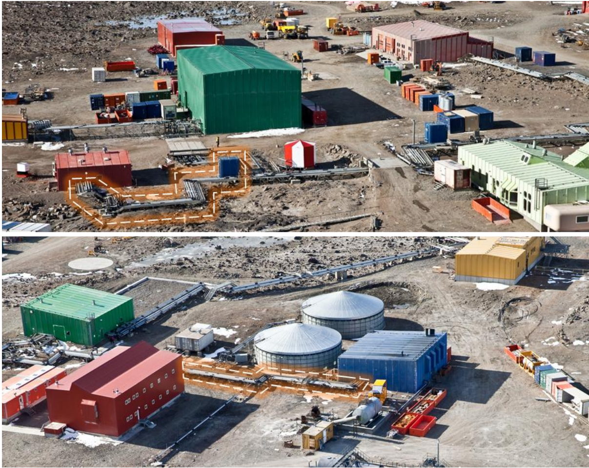
Figure 27. Davis station Emergency (top) and Main (bottom) Powerhouse service reticulation infrastructure flagged for removal (orange border) (Photo credit: David Barringhaus 2012)
