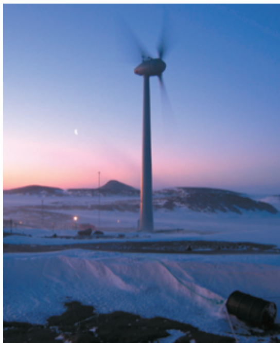
Wind turbines now provide up to 80% of Mawson station's power requirements.
