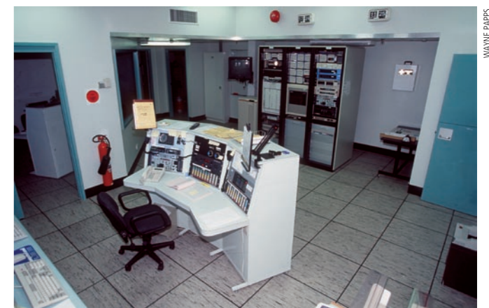
Communication technology has come a long way since the days of Mawson's 1911-14 expedition when a rotary-arc transmitter and Morse code were used to send weather information and personal messages (top). Today the communications room at Mawson station (above) contains the main control console and associated equipment.
